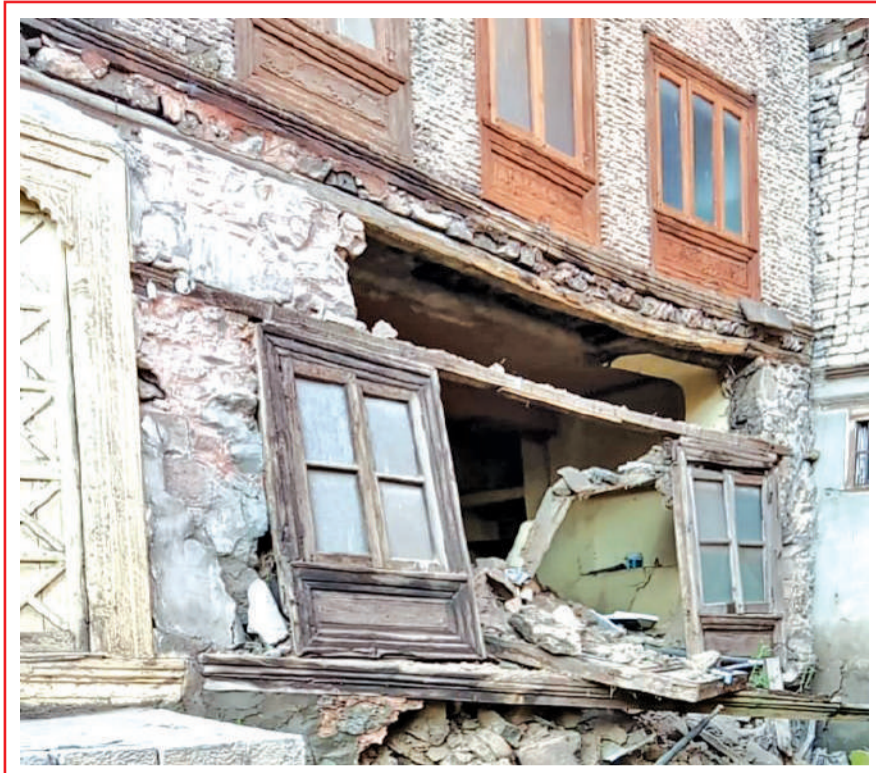
Inviting trouble, anytime can cave in. Residents of Hawal urge authorities to stop any tragedy.
